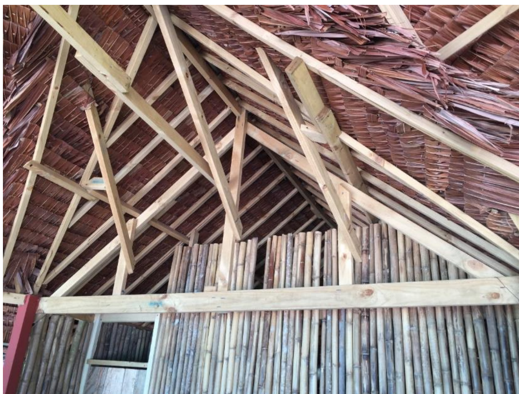
Figure 2-14 Use of New Zealand radiata pine in construction of beach resort on Santo
